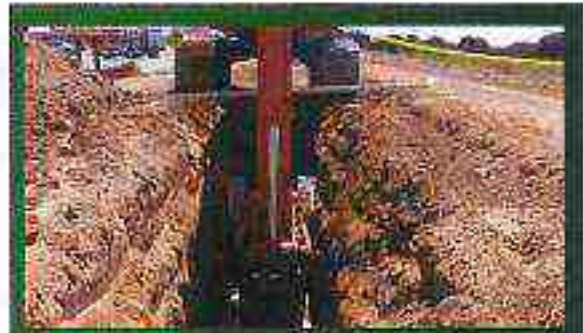
ACOG worked on the administration of an ARC grant to construct sewer lines along Highway 5.
